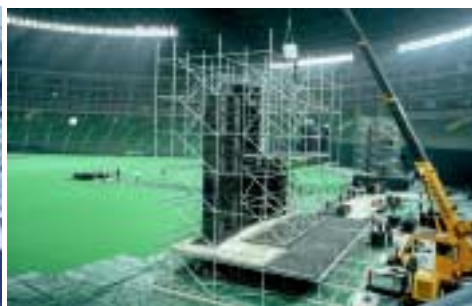
Fukuoka Dome Opening Ceremony '93 There was a certain presence of Rey Audio's clear and powerful sound right in front of people even in the troublesome environment in a dome.
